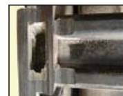
Links on the inner surface with no glide shoe attached (wear evident)
