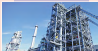
Biomass power plants Bucket elevators, conveyor chains
